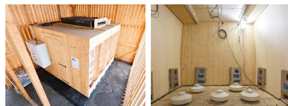
LIEBHERR's HVAC Subsystem with chamber
